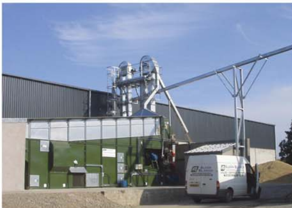
Commissioning of DF 30000 Drier
