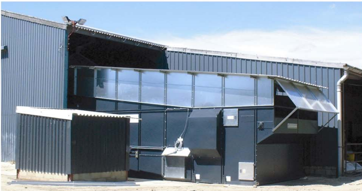
DF 30000 Drier - part external installation, blends well with modern buildings in keeping with tight planning constraints
