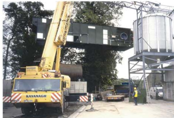
Main section of DF 42000 Drier - 47t/hr - lifted from truck to final position
