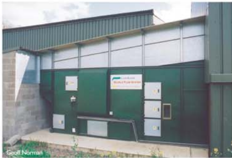
DF 17750 Drier - 19.5t/hr - with blockwork dust collection house at rear
